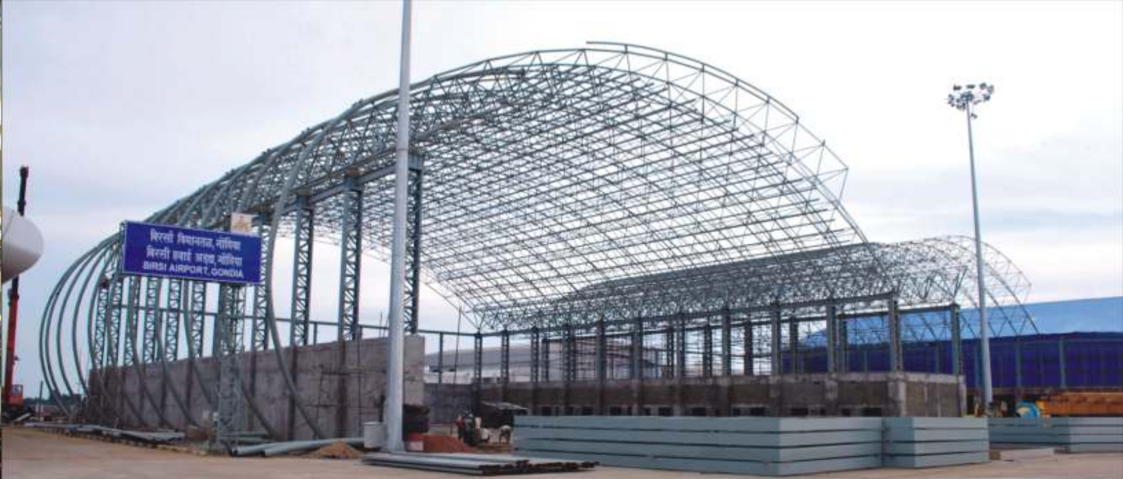
Gondia Airport Hangar, Gondia A unique shaped spaceframe structure covering an area of 9000 sq. ft. with a working height of 21 mtrs.
